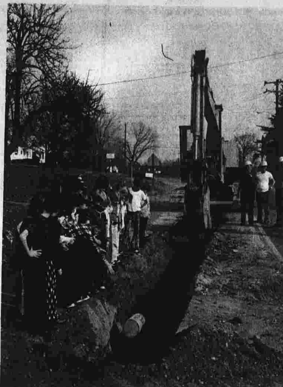
Fourth grade students of Buckland School and construction workers watch Michael Masse as he throws a time capsule prepared by the class into the ditch being dug for a new water main on Tolland Tpk. near the junction of N. Main St. For how long a time the capsule will remain there is anyone's guess. The water main to be installed is said to be a non-corrosive material. (Herald photo by Pinto)
